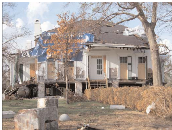
The storm spared nothing in its path, not even the former home of Jefferson Davis, the civil war Confederacy’s only president. The national historical landmark was seriously damaged.
