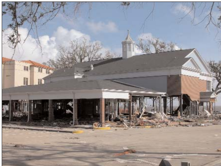
The depth and force of surge water from Katrina is registered on the brick walls of this funeral home across the street from the Gulf.
