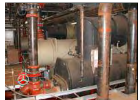
The casino boat's high end HVAC equipment will normally operate using 100 percent outside air.
